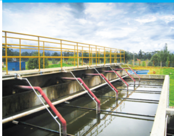
SISTEMA AIR-LIFTS RESIBLOC III 30 LPS PAIPA BOYACA
